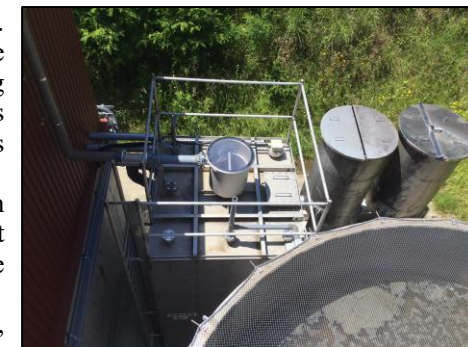
Kui Farm Compost Field Rainwater Storage Tank
